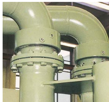
STENFLEX® Swivel Joints type DG-02S installed at loading arms
