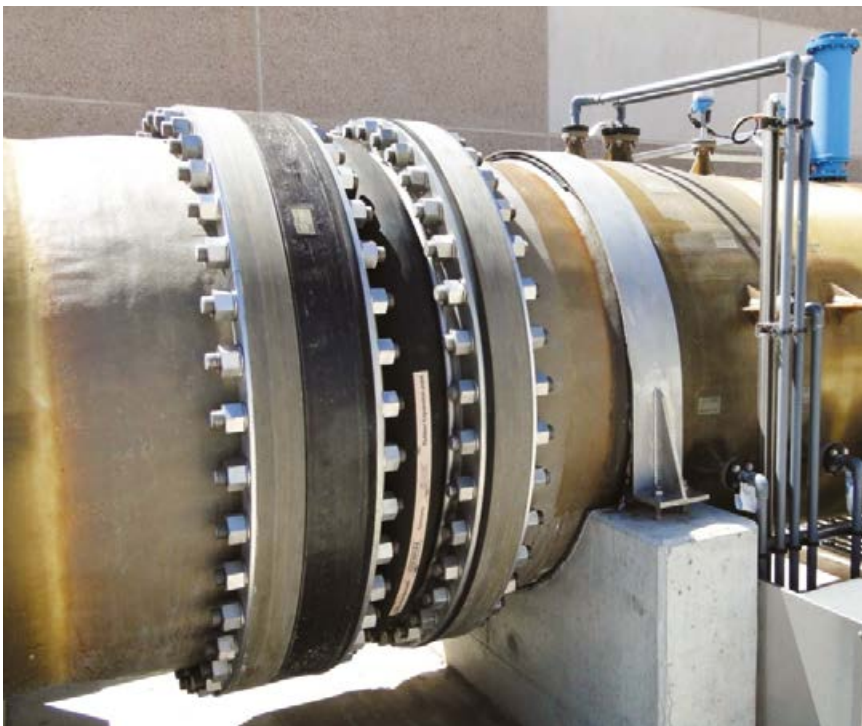
STENFLEX® offers regular inspections to ensure reliable plant operation
